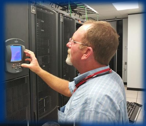
Thomas Hollister checking readings on CRAC unit A.
