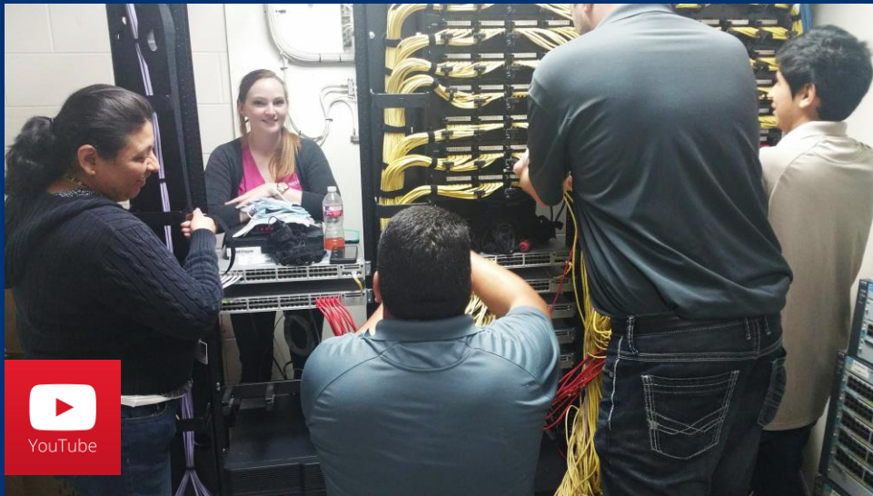
Anna Senties, Enterprise Communications Network Analyst with Presidio and Gigabit Contractors upgrading the main network electronics closet at Wilburn Elementary
