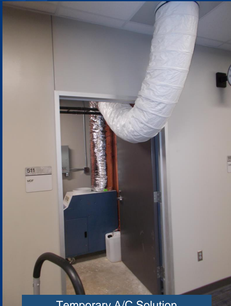
Temporary A/C Solution
