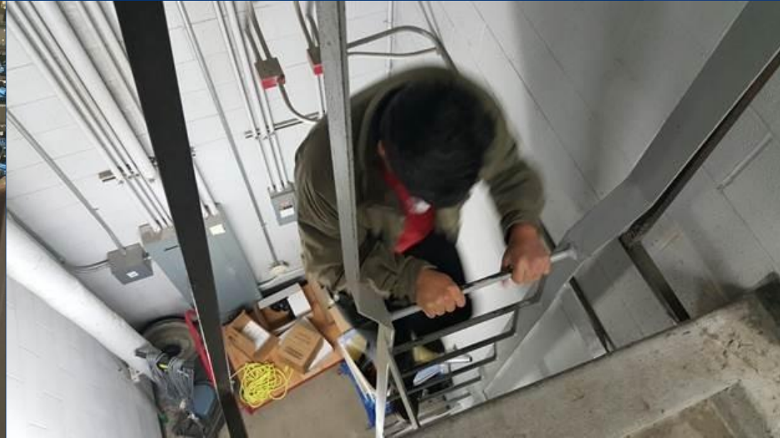
Walk through at Horne Elementary where IDF-C is above the gym and the only access is by way of a ladder
