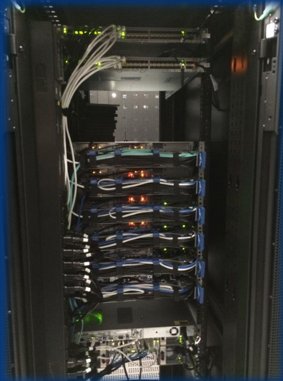
Point of Delivery (POD) for Network Services
