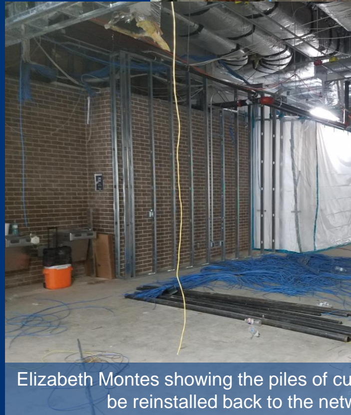
Elizabeth Montes showing the network closet rack and how all equipment is protected
