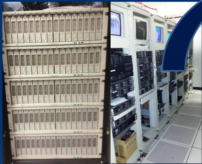
1990 Data Center Technology with Individualized Servers and Tape Backups
