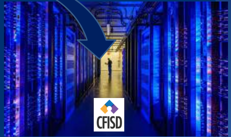
2016 Data Center Technology with a Virtualized Platform and High-Speed, Flash Array with Dual Backups
